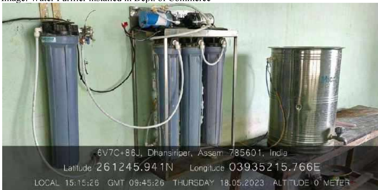
Image: Water Purifier Installed in Girls' Hostel
